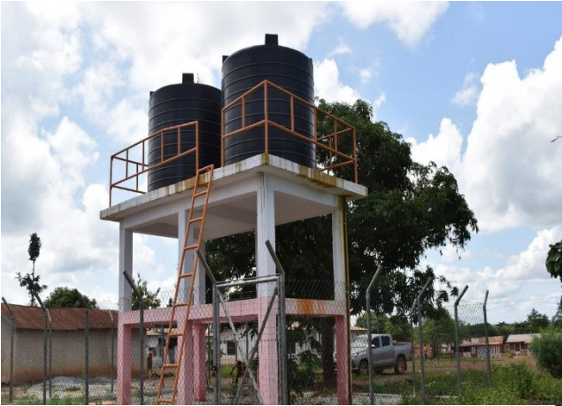
☐ SOLAR POWERED BOREHOLE AT KOJO NKRUMAH
