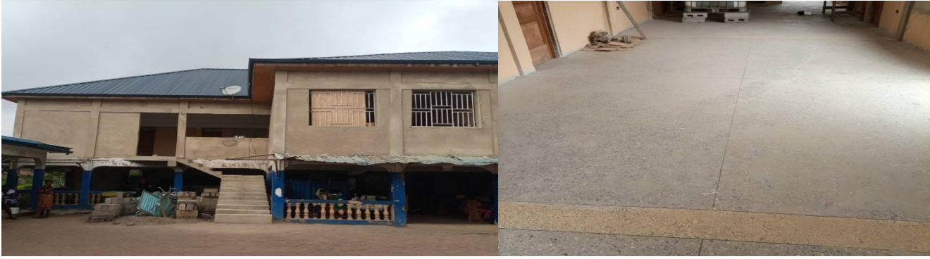
10. Construction of ENT room, consulting room and offices as first floor and redevelopment of the ground floor of Prestea Government Hospital
