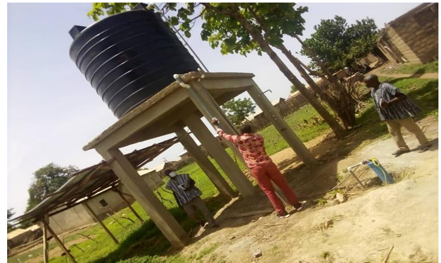
Hain Market Hand Washing Facility (Water Tank)
