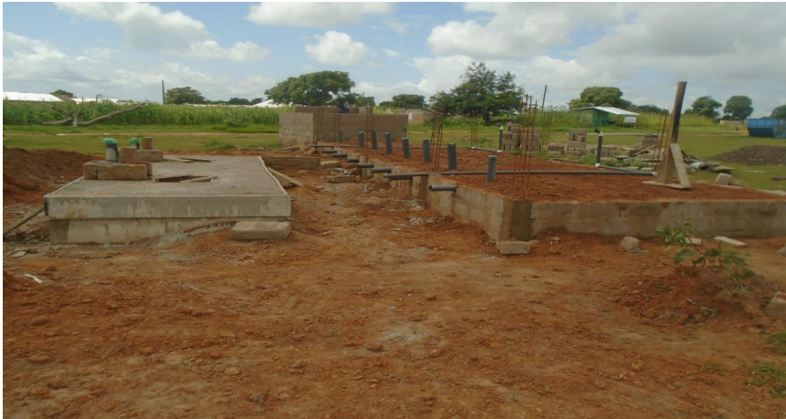
PROJECT: Construction of 1 No. 6 Unit Pour flush WASH Facility Nyosbara Funding Source: DACF-RFG STATUS: Floor Level
