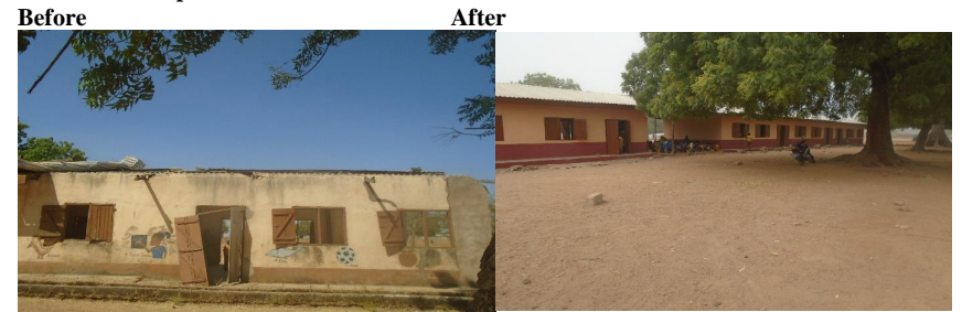
PROJECT: Renovation of 1No. 6 Unit classroom block at Kongo, Sabzunde, Bulpelsi, and a Teachers Bungalow at Kulbore. Funding Source: DACF STATUS: Completed and in use
