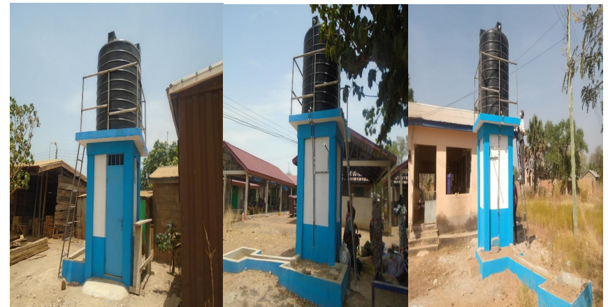
Drilled and mechanized 3no. Boreholes at Timber Market, Zuarungu Market and Gambigbo CHPS (COVID-19)
