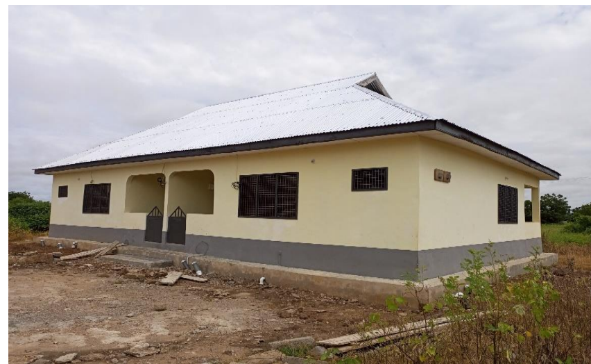
Construction and furnishing of 1No. Semi-Detached Bungalow for the Municipal health services in Yendi
