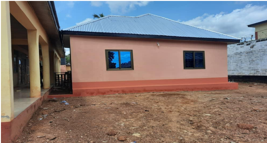
Construction of additional 1No. 3-units Office block with wash rooms at Yendi District Court.
