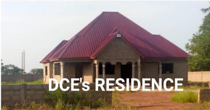
1. Construction of DCE's Residence with an Outhouse and a Fence Wall- (DA CF)
