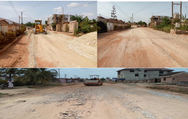
RE-SHAPING AND SPOT IMPROVEMENT OF ASHONGMAN PURE WATER ROAD (GOLD AVENUE RD)
