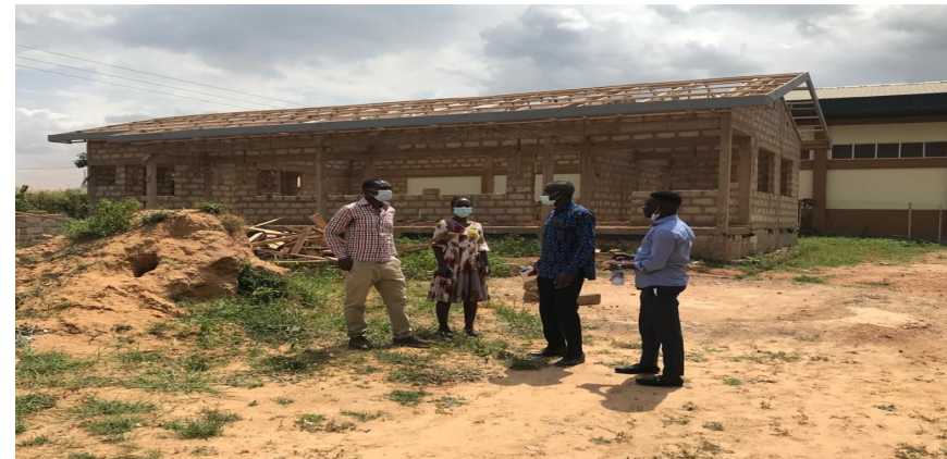
CONSTRUCTION OF ADMINISTRATION BLOCK, HATCHERY, PROCESSING CENTRE AS PART OF FIDEP PROJECT (PHASE II) 70% COMPLETED
