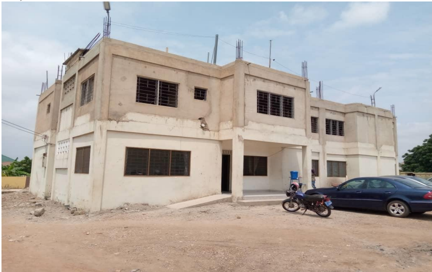
CONSTRUCTION OF 1 NO. 4-STOREY SUTSURUNAA ZONAL COUNCIL OFFICE BLOCK (PHASE II) 85% COMPLETION
