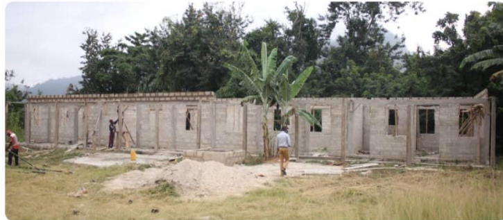
CONSTRUCTION OF 1 NO. 6 UNIT CLASSROOM BLOCK AT OBAWALE L/A PRIMARY SCHOOL – DACF RFG - (51 % COMPLETED)
