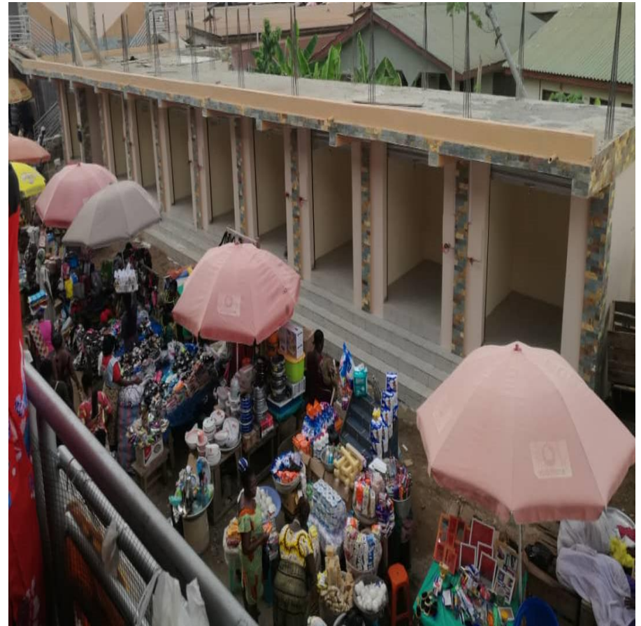
This constructed 12-unit lockable stores is a wholly funded from District Assembly Common Fund-Responsive Factor Grant (DACF-RFG) project and was completed within schedule and it's in use. This is aimed at further boosting the local economy of the municipality.
