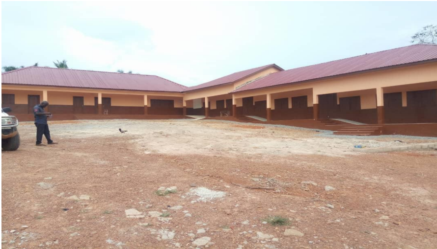
Construction of 1No 3-unit Class Room Block, Store, Library, Office with 6- seater KVIP Toilet and 4 urinals at Onyinafonsu
