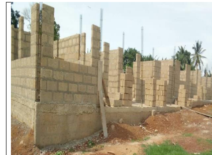
Construction of 1No. 3-Unit Classroom Block, Urinal, KVIP and Office at Kwahu Tafo. (35% Completed)
