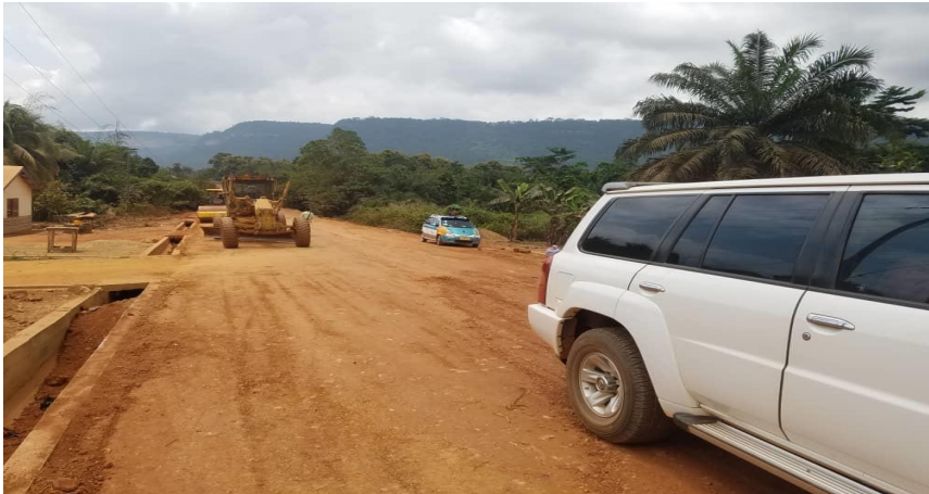
CONSTRUCTION OF 16.0KM ROAD FROM AKYEM OSINO TO AKYEM BOSUSO (FUNDED BY GoG) – 45% COMPLETE
