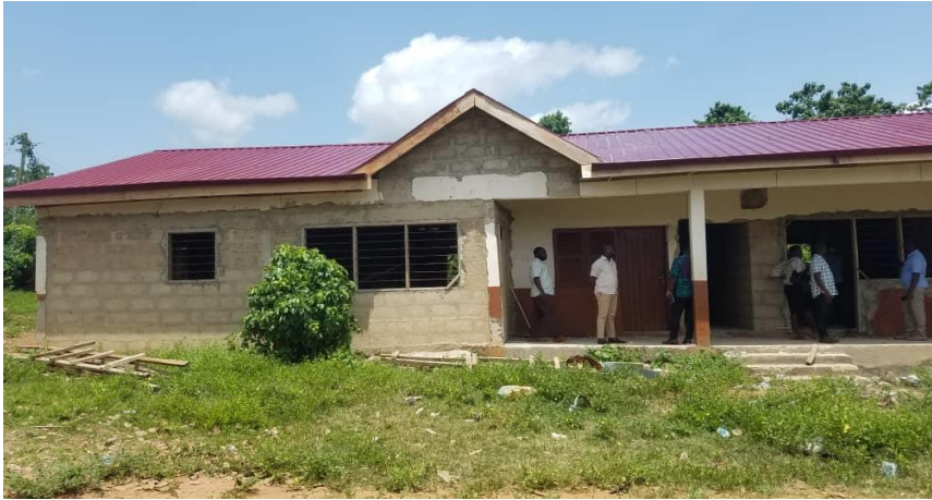
Conversion of 3-Unit Classroom Block into CHPS Center at Bepoase (Funded By: DACF) – 55% Complete
