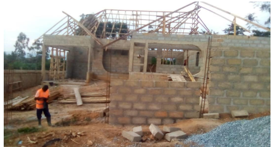
Construction of 1No. 4-Bedroom Magistrate Bungalow at Akyem Osino (Funded By: MLGRD) – 65% Complete
