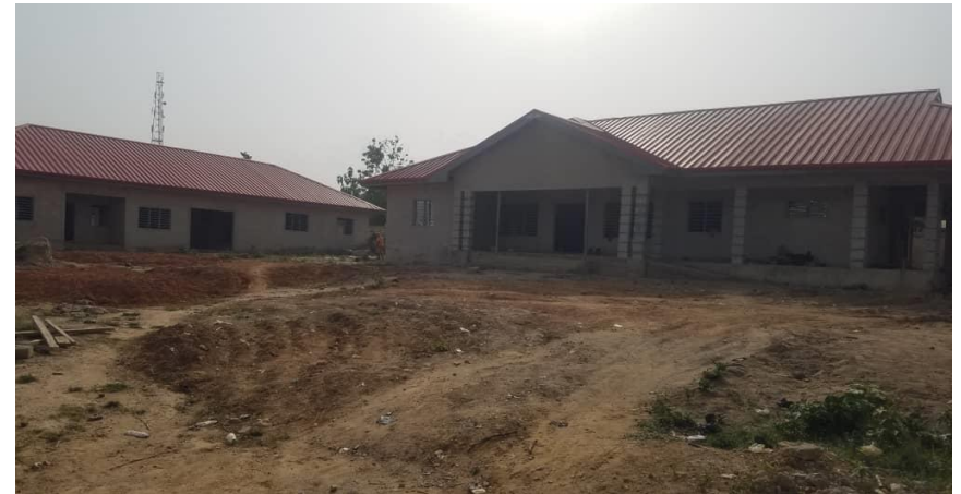
Construction of Health Facility with Nurses' Quarters at Akyem Nsutam (Funded By: MoH) – 75% Complete
