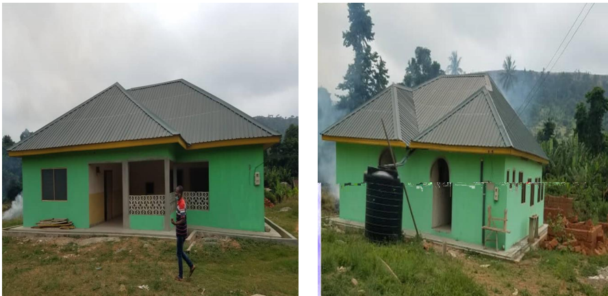
CONSTRUCTION OF 1NO. CHP COMPOUND AND NURSES' QUARTERS AT ASEDJA AKWADUM (FOUNDED BY DACF) – 95% COMPLETE
