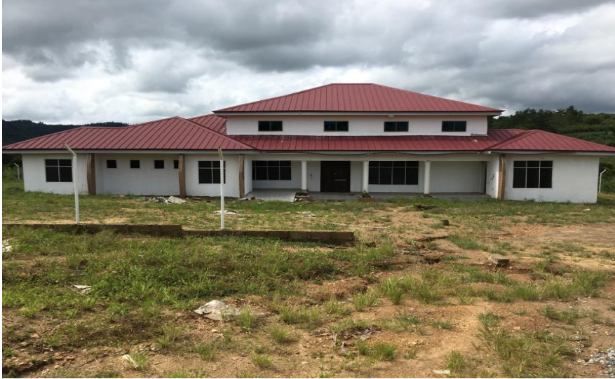
Constructed 1No. Single Court Complex for the Ayensuano District Assembly at Coalta.
