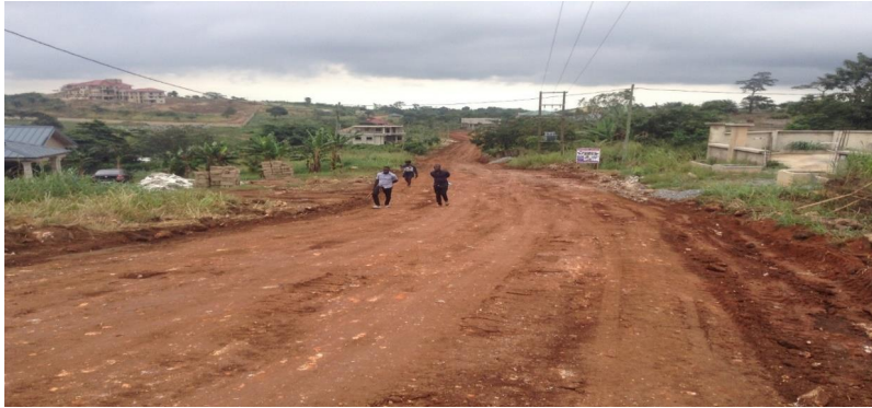
GRADING / GRAVELLING AND RESHAPING OF 5KM ROAD NETWORKS WITHIN AKROPONG AND ITS ENVIRONS
