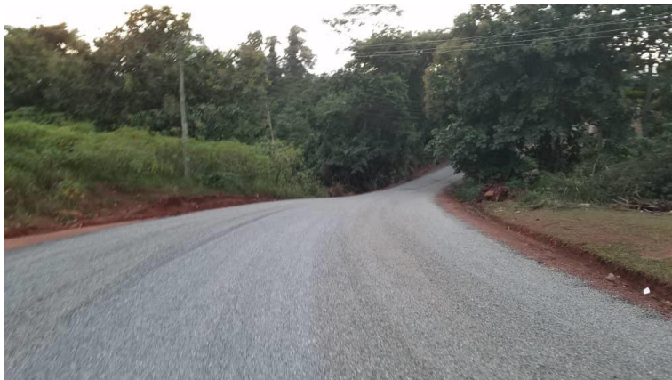
SEALING (BITUMINOUS SURFACING) OF OFFICE ROAD FOR AKUAPEM NORTH MUNICIPAL ASSEMBLY, AKROPONG – 0.35KM
