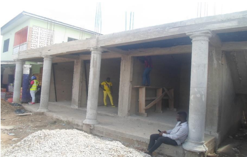
Construction of 1 No. 3 Unit Trading store at Breman Breman Asikuma Phase 1 with IGF
