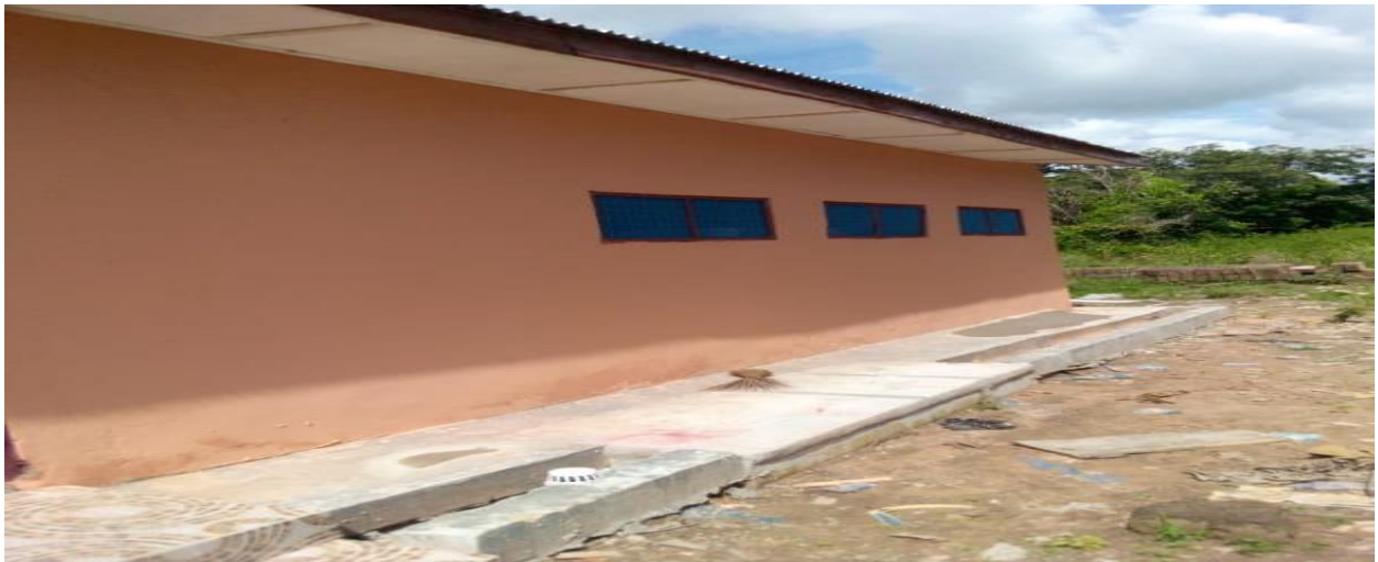
1 NO 10 Seater WC Toilet Facility at Fumsua
