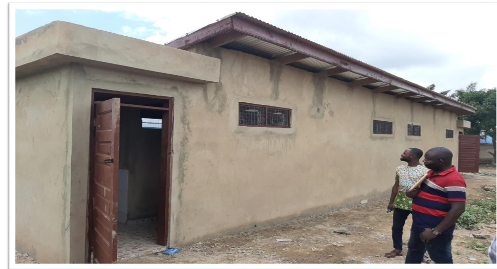
1NO. 10SEATER W/C UNDER CONSTRUCTION AT DAMANKO YAM MARKET (FROM INTERNALLY GENERATED FUND –IGF)
