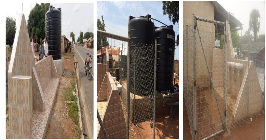
Figure 4: Rehabilitation of Small Eath Dams at Wulensi and Nakpayili & Hand Washing Facilities constructed at Nakpayili,Wulensi and Lungni
