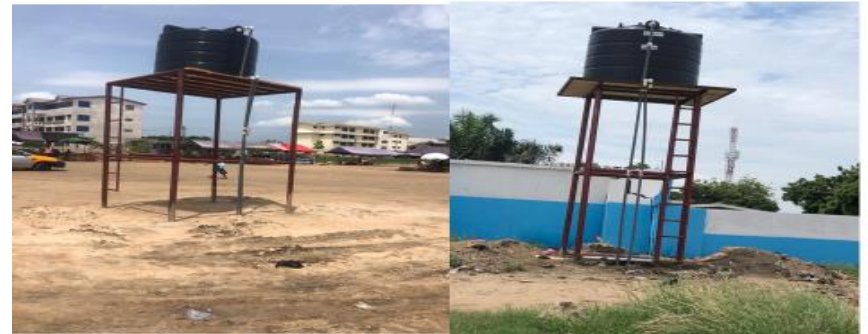
Construction of pipe borne water at various Markets to promote hand washing and hygiene to fight COVID 19
