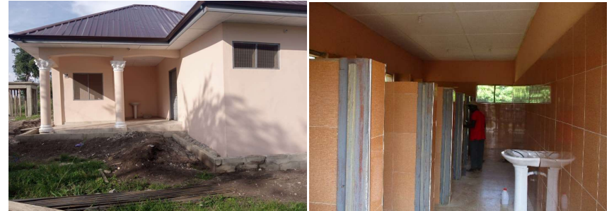
Completion of 2No. 14 Seater W/C toilets, water system and Biogas at Abetifi Technical Institute and St. Joseph Technical Institute at Kwahu Tafo
