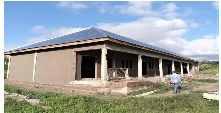
1NO 3-UNIT CLASSROOM BLOCK STAFF COMMON ROOM, LIBRARY & STORE AT AKRUMA CONSTRUCTED AT ROOFING LEVEL
