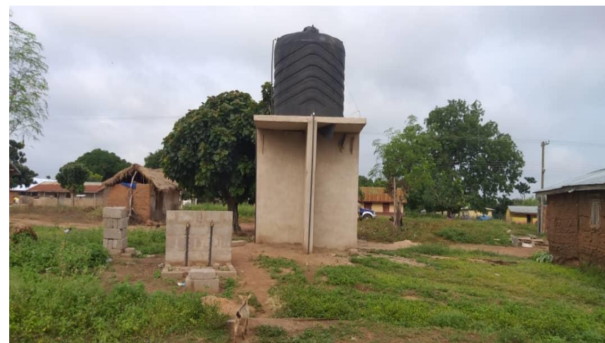
MECHANIZATION OF 7NO. BOREHOLES AT NANTE, AGYEGYEMAKUU ,APESIKA ,AKORA, MANSIE, PUMPUATIFI AND FORIKROM
