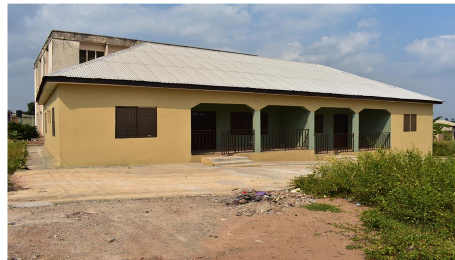
Construction of 1No. 2 Bedroom Semi-Detached Staff Bungalow at Mamponteng in Kwabre Municipality
