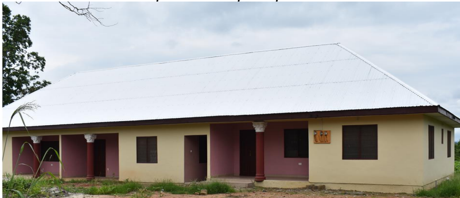
Construction of 1No. 3 Unit 2 Bedroom Teachers Quarters at Amanpe in Kwabre East Municipality
