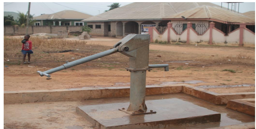
BOREHOLE FITTED WITH HANDPUMP AT YAW NKRUMAH
