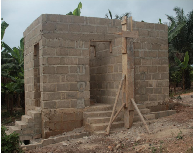
4-SEATER WC- AND 2-URINAL FACILITY WITH A MECHANISED OVERHEAD TANK FOR ACHIASE HEALTH CENTRE
