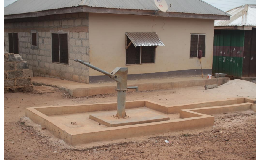
BOREHOLE FITTED WITH HAND PUMP-NEW BOMFA
