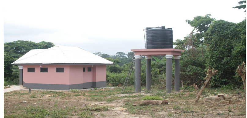
5-SEATER WC AND 2 URINAL FACILITY WITH A MECHANISED OVERHEAD TANK AT BOMFA HEALTH CENTRE
