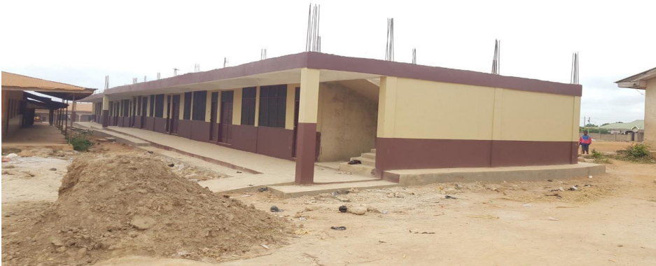
CONSTRUCTION OF 1 NO. 6 UNIT CLASSROOM BLOCK WITH OFFICE AND STORE AT APUTUOGYA D/A PRIMARY
