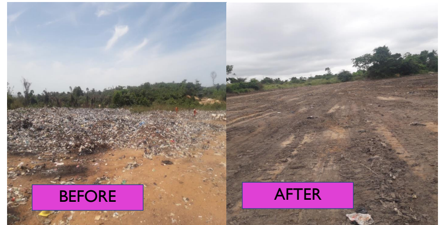
i). REFUSE EVAQUATED AND LEVELLED AT FINAL REFUSE DISPOSAL SITE AT SESEKRO.
