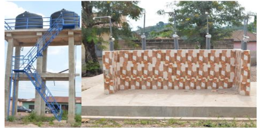
COMPLETED 1 NO. MECHANIZED BOREHOLE AT PATRIENSA IN THE ASANTE AKIM CENTRAL MUNICIPAL
