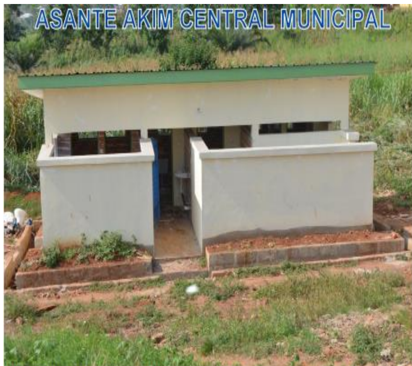
ON- GOING CONSTRUCTION OF 6 SEATER TOILET FACILITY FOR GIRLS LOCATION: KONONGO ODUMASE SENIOR HIGH SCHOOL GPS ADDRESS; AC- 0039- 8282
