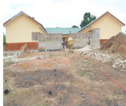
ON- GOING CONSTRUCTION OF 6 UNIT CLASSROOM BLOCK AT ABOSOMTWEAGYA GPS ADDRESS: AC-0024- 0520
