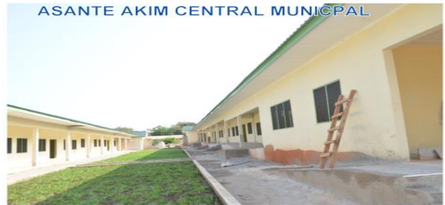
ON-GOING SINGLE STOREY DORMITORY BLOCK LOCATION: KONONGO ODUMASE SENIOR HIGH SCHOOL GPS ADDRESS: AC- 0039- 8282
