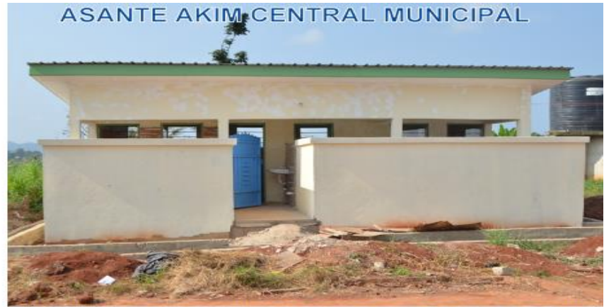
ON- GOING CONSTRUCTION OF 6- SEATER TOILET FACILITY FOR BOYS LOCATION: KONONGO ODUMASE SENIOR HIGH SCHOOL GPS ADDRESS: AC- 0039- 8282
