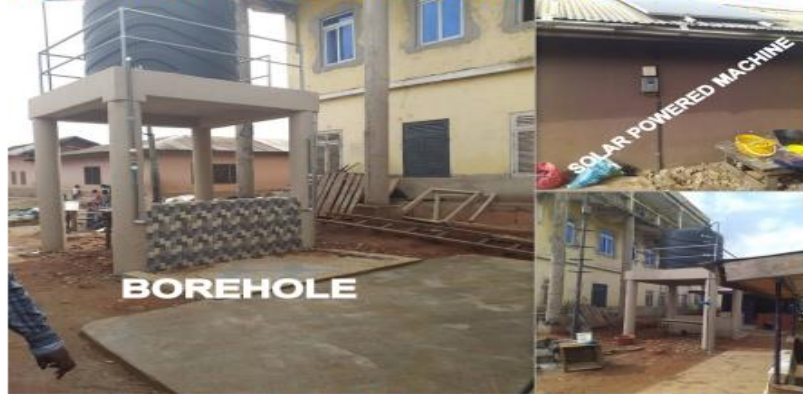
PROJECT TITLE: CONSTRUCTION OF 1 NO SOLAR POWER MECHANIZED BOREHOLE LOCATION: KONONGO- AHENBRONUM SOURCE OF FUNDING: YMCA STATUS: COMPLETED
