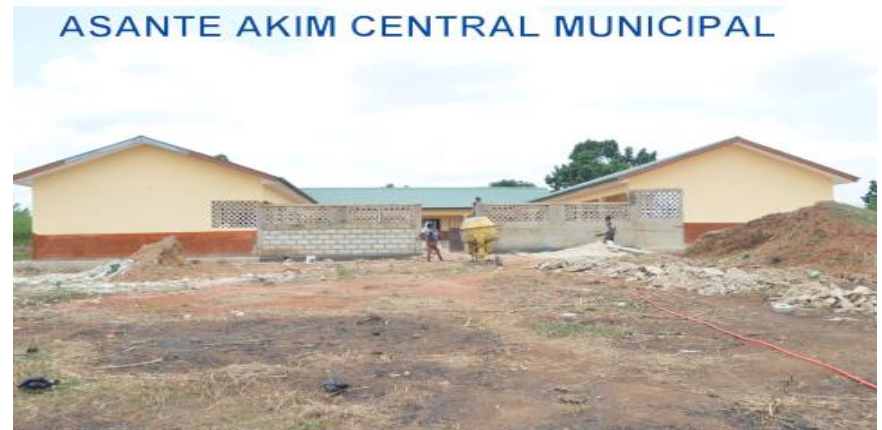
ON- GOING CONSTRUCTION OF 6 UNIT CLASSROOM BLOCK AT ABOSOMTWEAGYA GPS ADDRESS: AC- 0024- 0920
