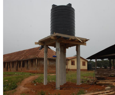
Construction and Mechanisation of 1No. Borehole with 10000 Liters Polytank, 2 Stand Pipes and Veronica Buckets at Pokukrom Market (Funded by: DPAT II)
