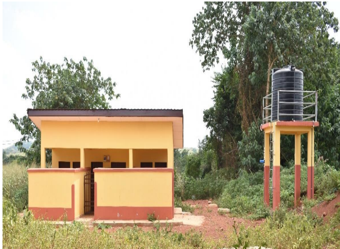
CONSTRUCTION OF 13NO. 6-SEATER WATER CLOSET WITH MECHANIZED BOREHOLE FACILITY IN THE MUNICIPALITY
