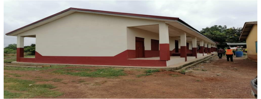
Construction of 1no. 6-unit Classroom block with Headmaster's Office at Gyamfi Kumanini SHS - Wamahinso
