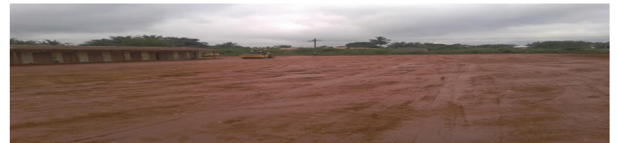
Construction of 1NO. 3unit classroom block for Odeniho Basic School at Kenyasi
