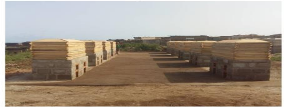
Project Description: Construction of improved “Ahortor” Oven at New Town, Bankuman Digital Address: GT-149-2112 Funding : CLGF
