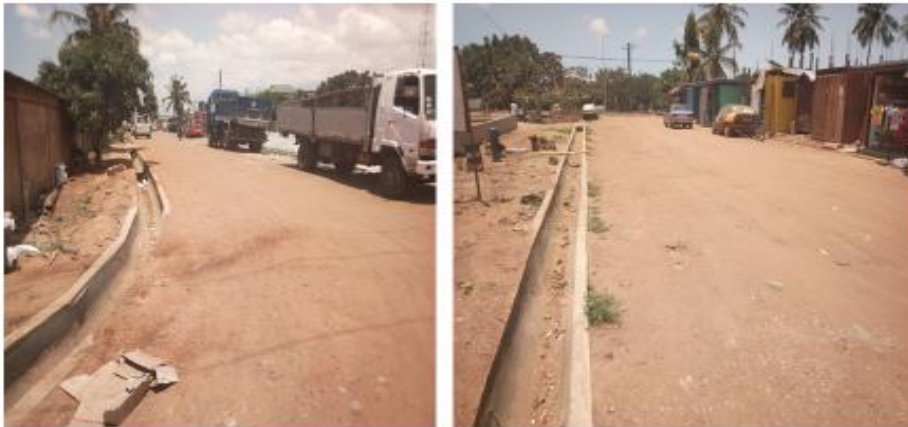
Project Description: Construction of U-drain and re-surfacing of 4.13 km road at Comm. 9 Digital Address: GT-217-3383
