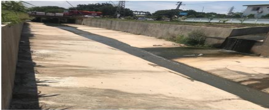
Project Description: Concrete storm drain at Comm. 6 Digital Address: GT-085-2161 Funding : GAMA
