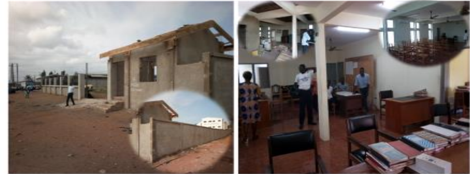
Project Description: Rehabilitation of Tema East Sub-Metro. Office Block Digital Address: GT-150-3102 Funding : DACF
