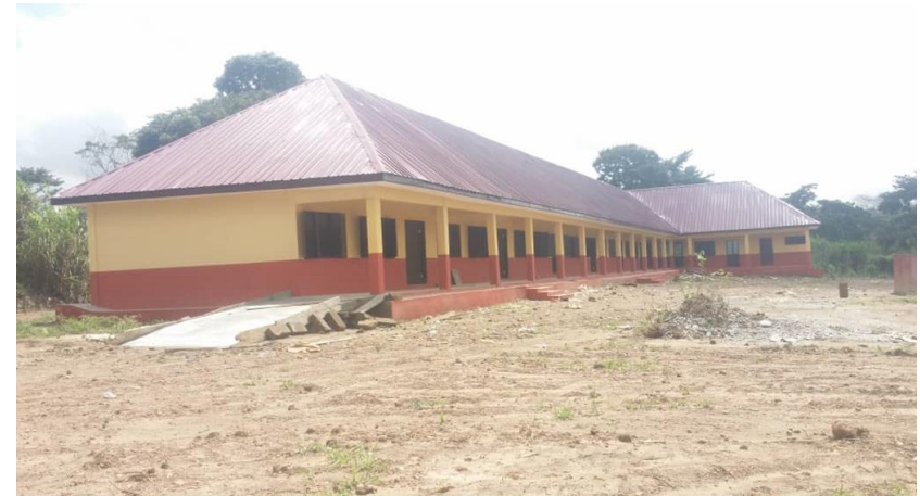
Construction of 6-Unit Classroom Block with Ancillary Facility for Fiapre Girls Model
