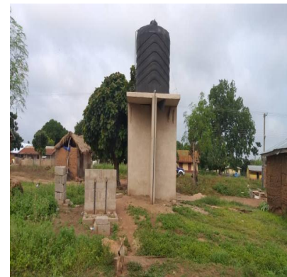
DRILLING, CONSTRUCTION, INSTALLATION AND MECHANIZATION OF 5NO. BOREHOLES ATAPAASO, KWABIA, PENINAMISA, SABULE AND BODWOM
