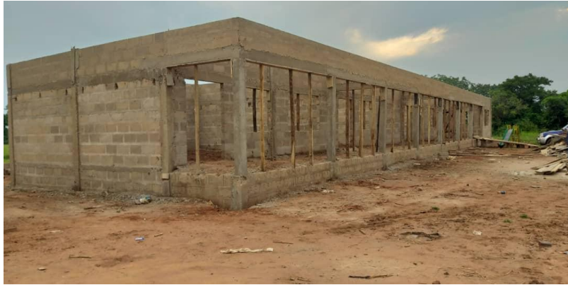
CONSTRUCTION OF 1NO 3-UNIT CLASSROOM BLOCK STAFF COMMON ROOM, LIBRARY & STORE AT BAABU
