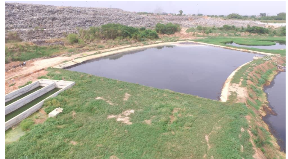
Figure 10: Ameliorated Anaerobic pond at Oti
