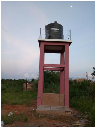
Figure 4: Mechanized Borehole With An Overhead Tank at Bantama
