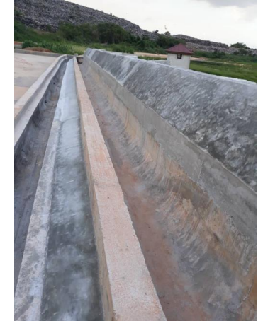
Figure 7: Headworks for faecal sludge discharging at Oti
