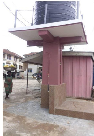
Figure 5: Mechanized Borehole With An Overhead Tank at Bohyen
