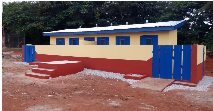
Construction of 1 No. 6-Seater KVIP toilet for Methodist Primary, Kenyasi No 2 Project Cost: GHc. 52,346.24
