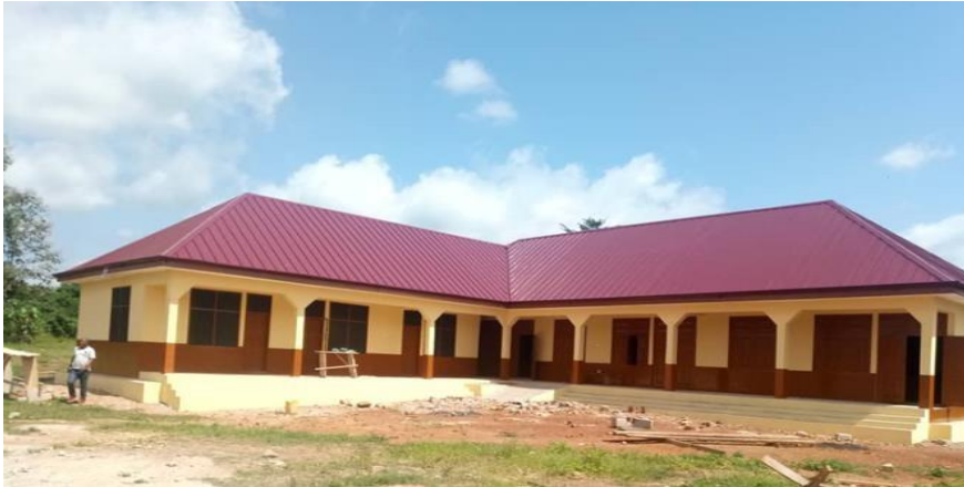
Construction of Single Storey 3-Unit classroom block with office, store, 4-unit KVIP, 2 Urinal and Change room at Tawiahkrom. Project Cost: GHc. 223,775.68
