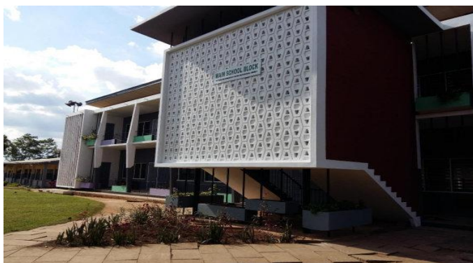
Renovation of 10 unit classroom Block at St. Louis Senior High School, Oduom
