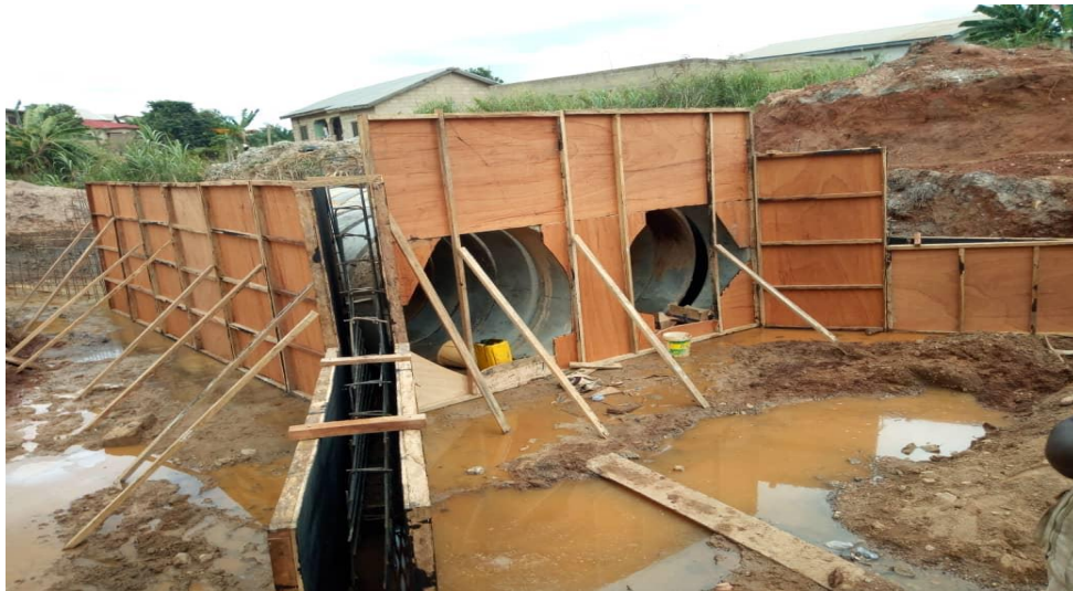
Project Name: Construction of District WAEC Depot Location: Kodie Funding Source: IGF
